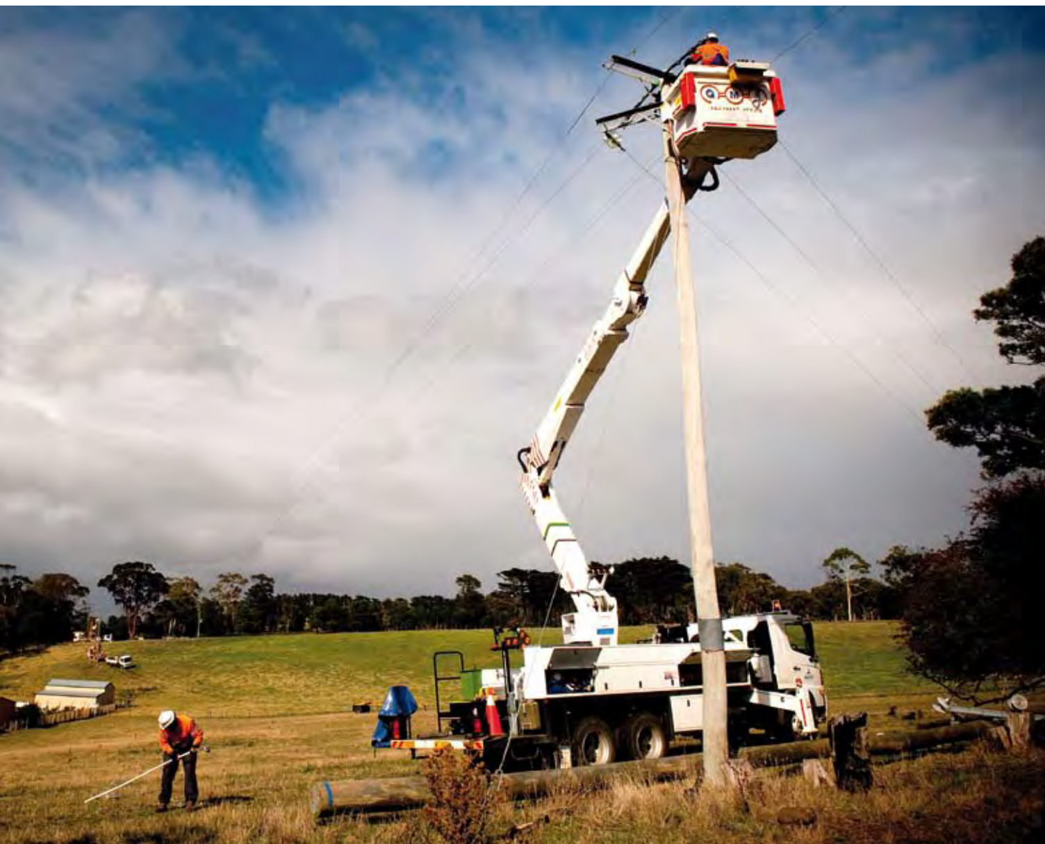
Crews came from all over the north to upgrade the power supply to the community of Clarence Point, near Beaconsfield, in April 2009.
