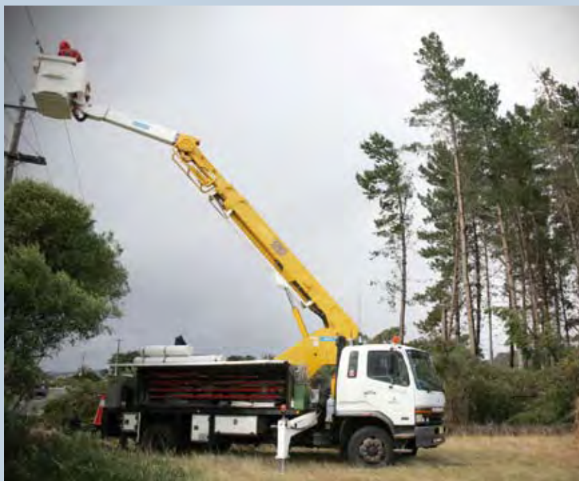
An Aurora crew repairs a pole damaged by lightning near Wynyard in April 2009.
