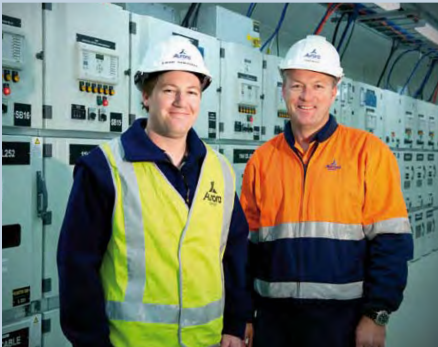
Graduate Engineer Ewan Sherman (left) and Project Manager Craig Wilson, inside the Cambridge substation.
