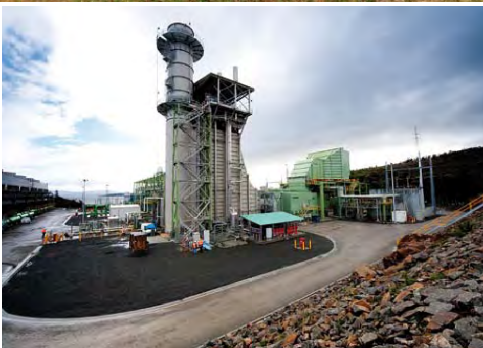
A view of the cooling tower (left), heat recovery steam generator (centre) and the Mitsubishi gas turbine (right) at the Tamar Valley Power Station.
